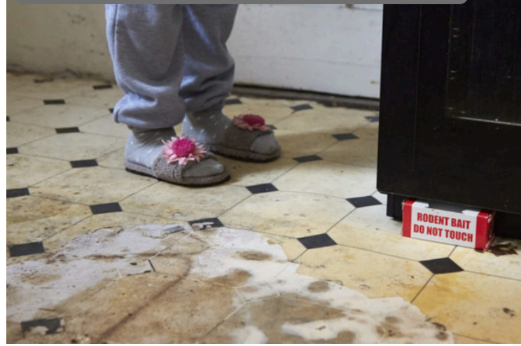
Image of home with mould and infestation
